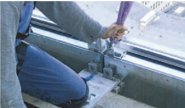
Fixing of a modular façade using HCW-ED Brackets on HTA-CE Cast-in channels
