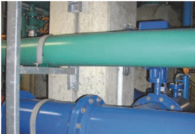
Pipe supports on vertical HZA Channels
