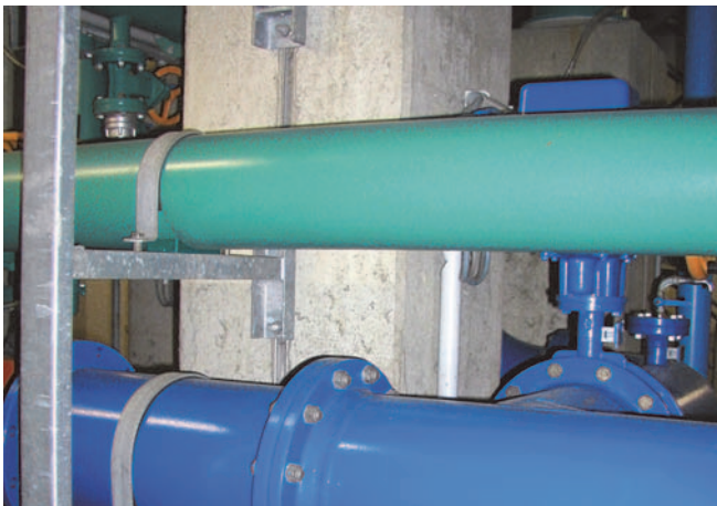
Pipe supports on vertical HZA Channels
